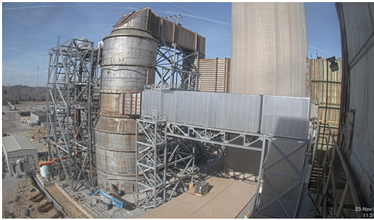
WILSON STATION SCRUBBER SYSTEM TO REDUCE EMISSIONS AND LOWER GENERATING COSTS
